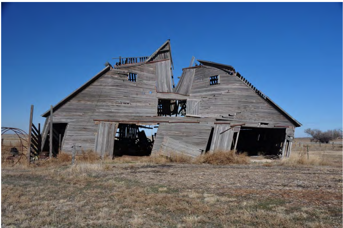
Landmark historic barn in ruins , Balko vicinity, Beaver County. This is the Blackwelder-Kinsey Barn, built in 1921. According to informants, it was constructed from the insurance settlement of an earlier barn lost to fire at the same location.
