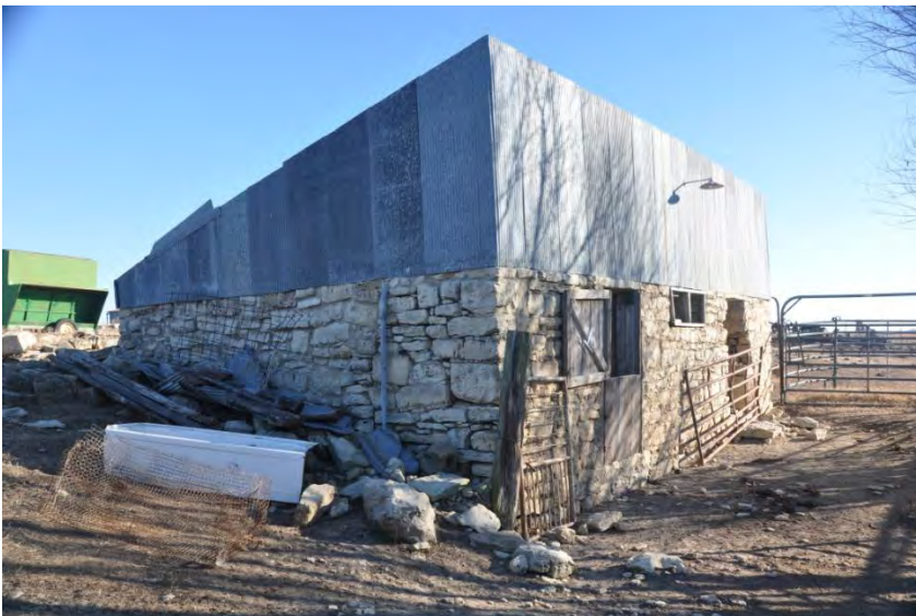
Ruins of Silverdale Stone Bank Barn , ca. 1947, Chilocco vicinity, Kay County. Originally this bank barn (above, painting) was gabled and used as a dairy barn. It makes use of the local limestone and is located only feet from the Kansas line. Having been leveled by a tornado, only the stone portion remains.
